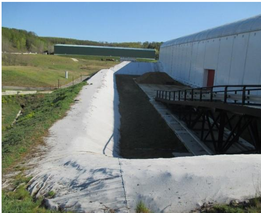
Fig. 11 The 2 nd stage of VLLW repository built next to the overlay hall of the operated 1 st stage of the VLLW repository after its relocation in 2019
