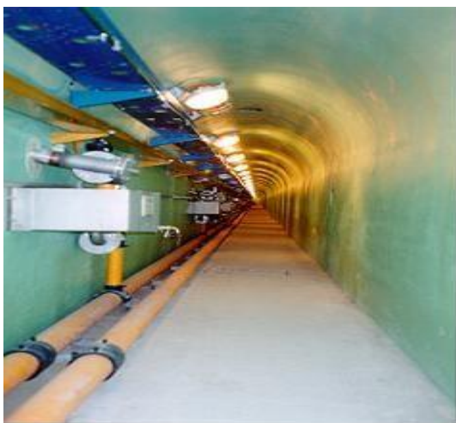
Fig. 26 Monitoring equipment at the National Repository of RAW
