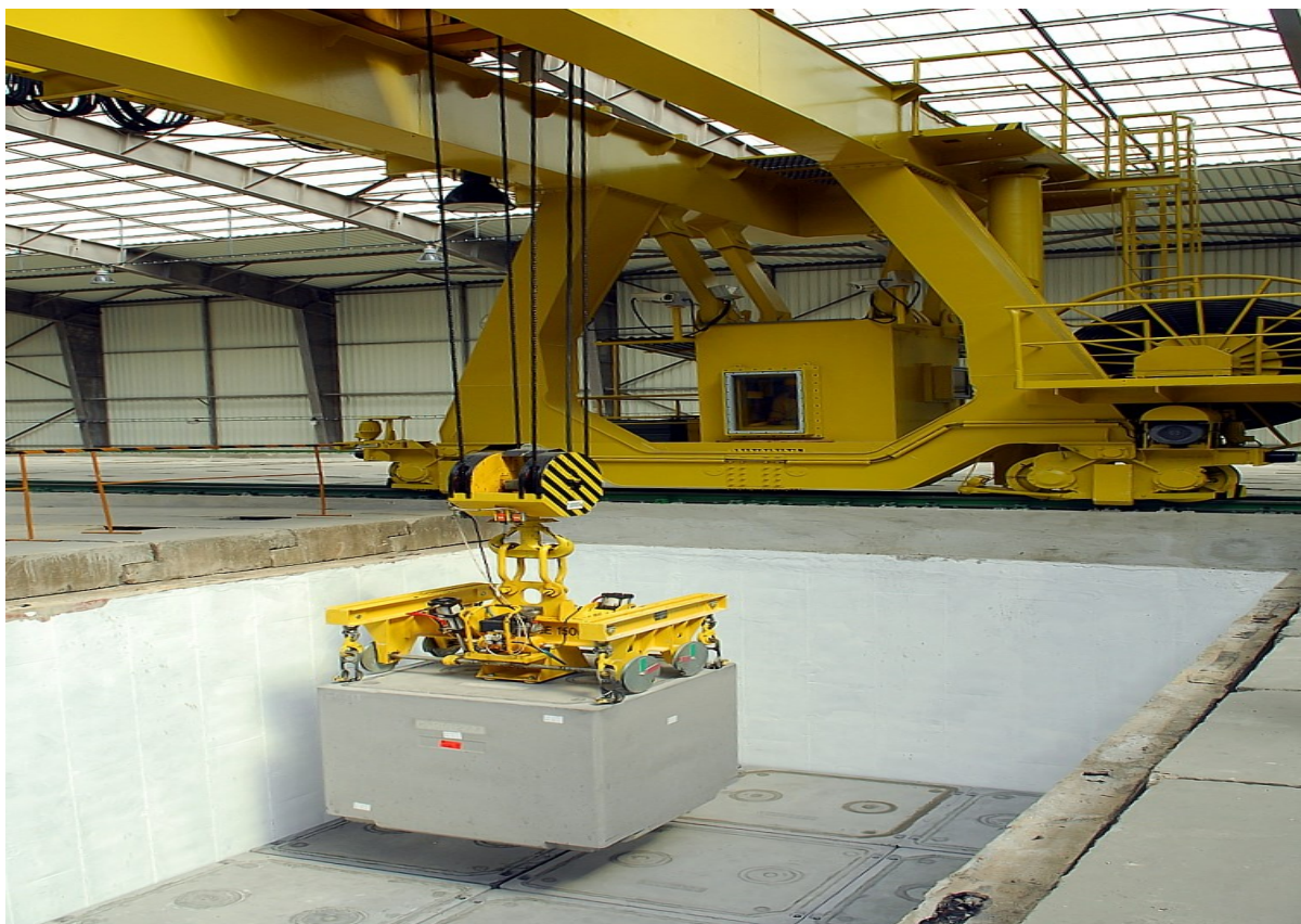
Fig. D.2.7a) VBK after measurements taken at Gamma scanner prior to disposal into disposal boxes of the repository arranged as double-rows
