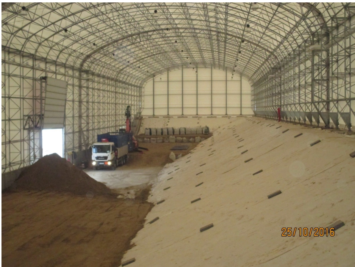
Fig. D.2.7b) Disposal of VNAO in the first stage of VNAO repository with a disposal capacity of 20 000 m 3 for RAW from the decommissioning of NPP A 1
