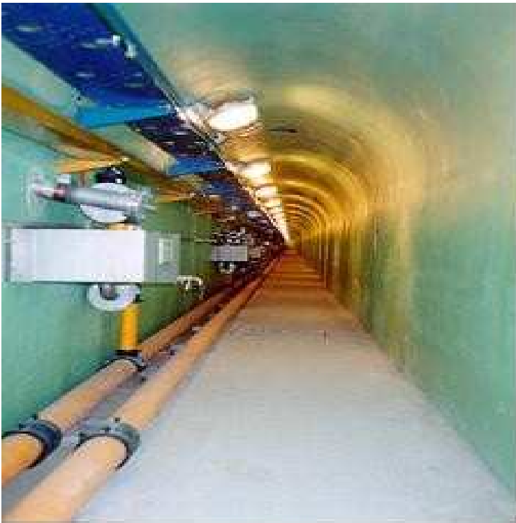
Monitoring equipment at the regional RAW repository
